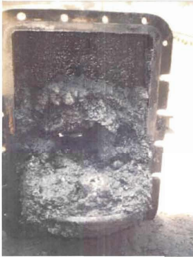
Fig. 13 Conventional Gooseneck Plugged by Tar
